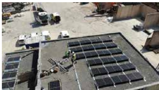
Solar Panels installed at Suttle Stone Quarries' Swanworth Quarry workshop.
