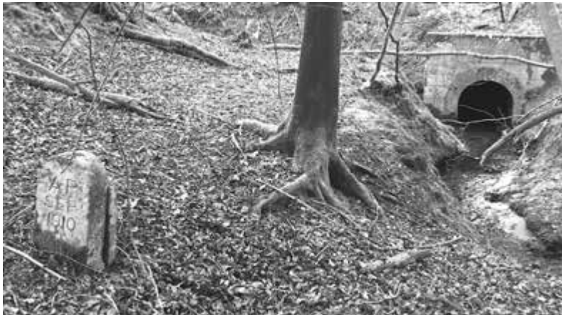
Photo of the western side of the railway line which crosses over the culvert for the Hixlade stream.
